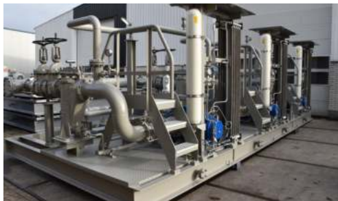
Crude oil pumps
