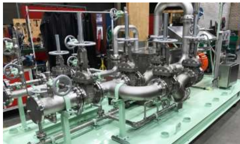
Water injection pump
