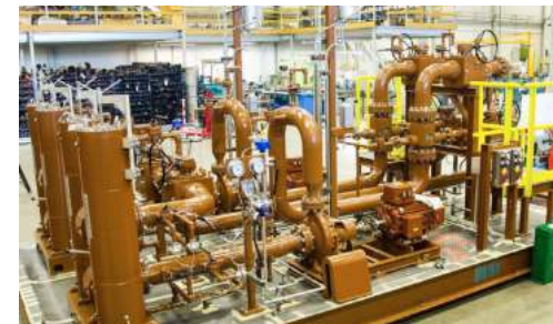
Fuel forwarding pumps
